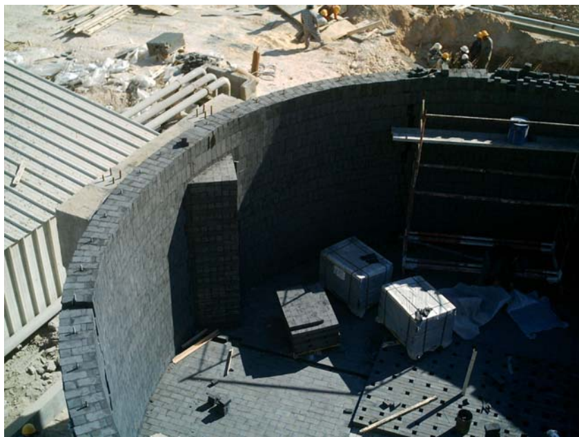
Rubber- and Brick-Lining for a concrete Reactor in the Filtration unit
