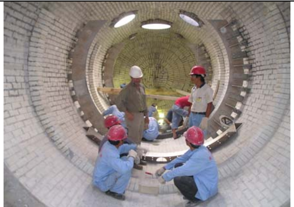
Brick lining in Autoclaves
